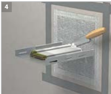
4 Mask the aperture 2 cm bigger than the aperture size, fill all remaining spaces with ROKU® MFC 100 coating.
